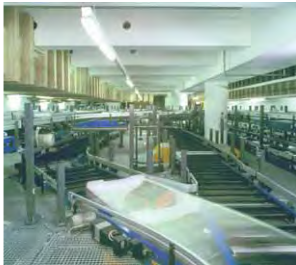
Figure 3. Snapshot into a BHS with a moving tote in the foreground
